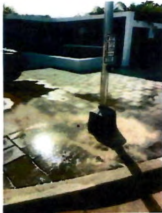
broken mainline landmark main entrance
