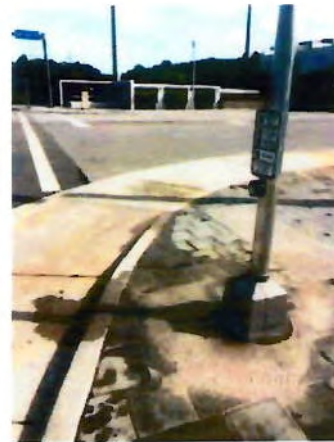
mainline break underneath pavers
